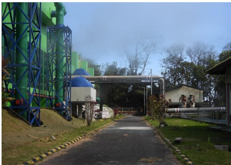
Gambar 9. Area Cooling Tower [Dokumentasi Tim, 2024]
